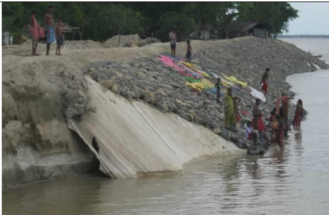
Photo 2: This embankment was made to prevent erosion at Village Madanpara downstream of Farakka on left bank. The embankment was itself eroded within one month of being made.
